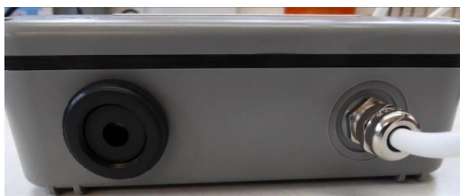
Speaker and cable to Beacon
